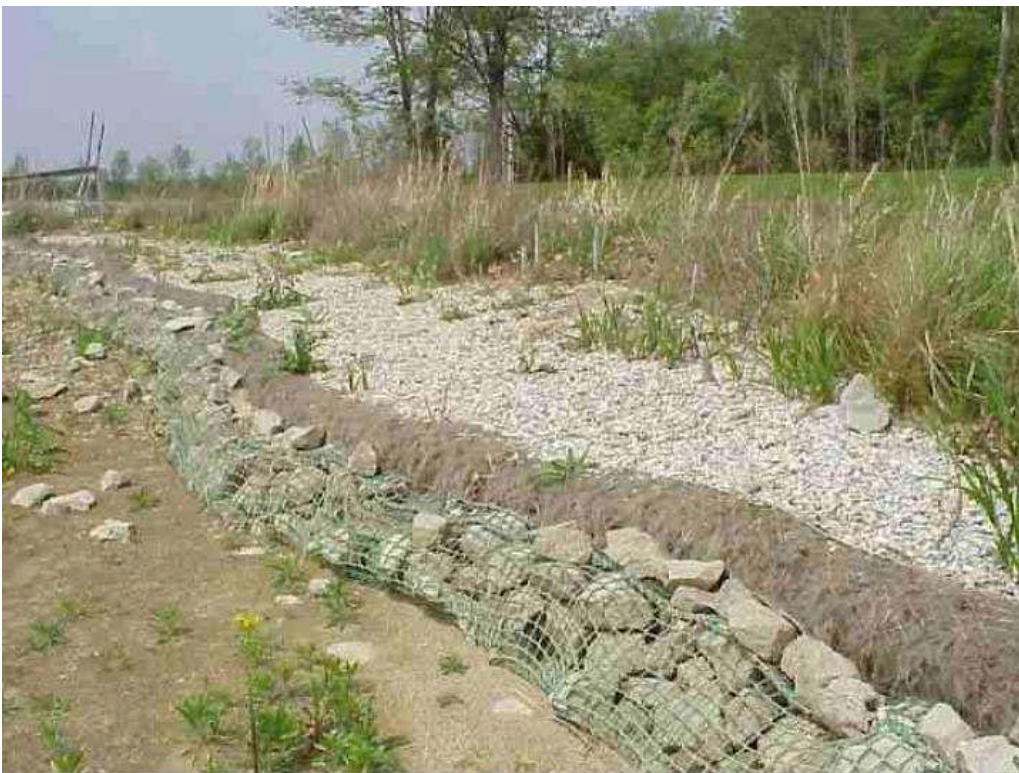
Photograph 4. Construction phase example of erosion control system that includes coir logs, riprap and vegetation.
